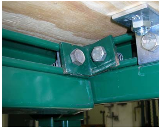
Figure 36: Deformed connection of spandrel girder under full water load
