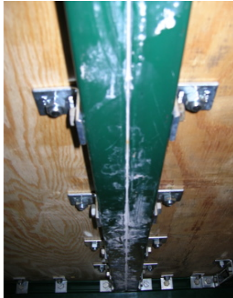
Figure 22: Double UNISTRUT ® supporting two sheets of plywood.
