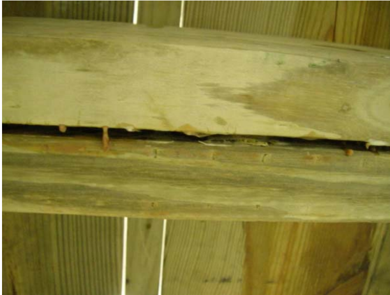
Figure 10.3: Gaps on the Bottom of the Central Girder due to Warping
