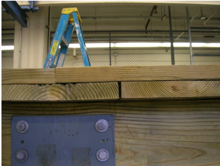
Figure 10.11: Opposing Grain Orientations on Deck Could Lead to Cupping and Ponding
