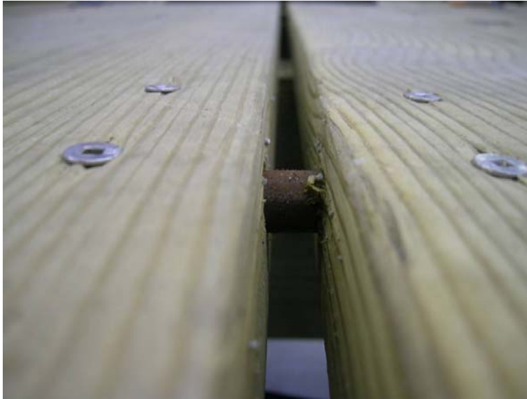
Figure 10.10: Shrinking of Green Deck Planks Exposing Gaps
